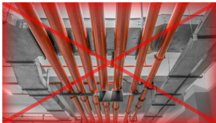
Figure 64 – sample unacceptable fire pipeline designation
