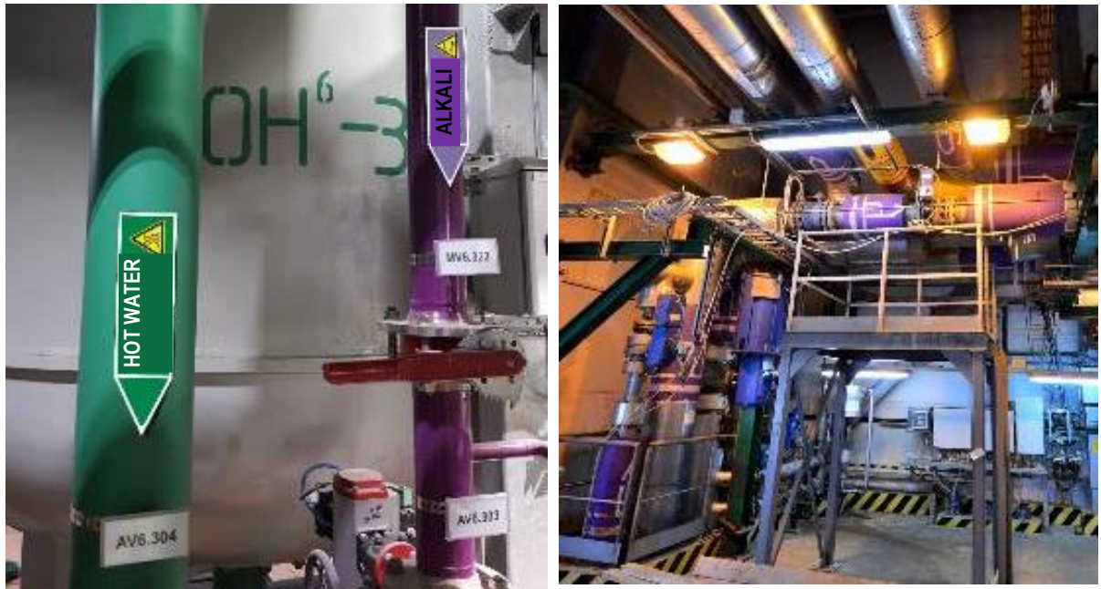
Figure 100 – sample application of identification paint on pipelines
