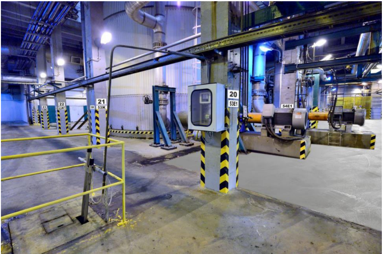
Figure 38 – sample application of color design of a number of piers, supports of the inner premises
