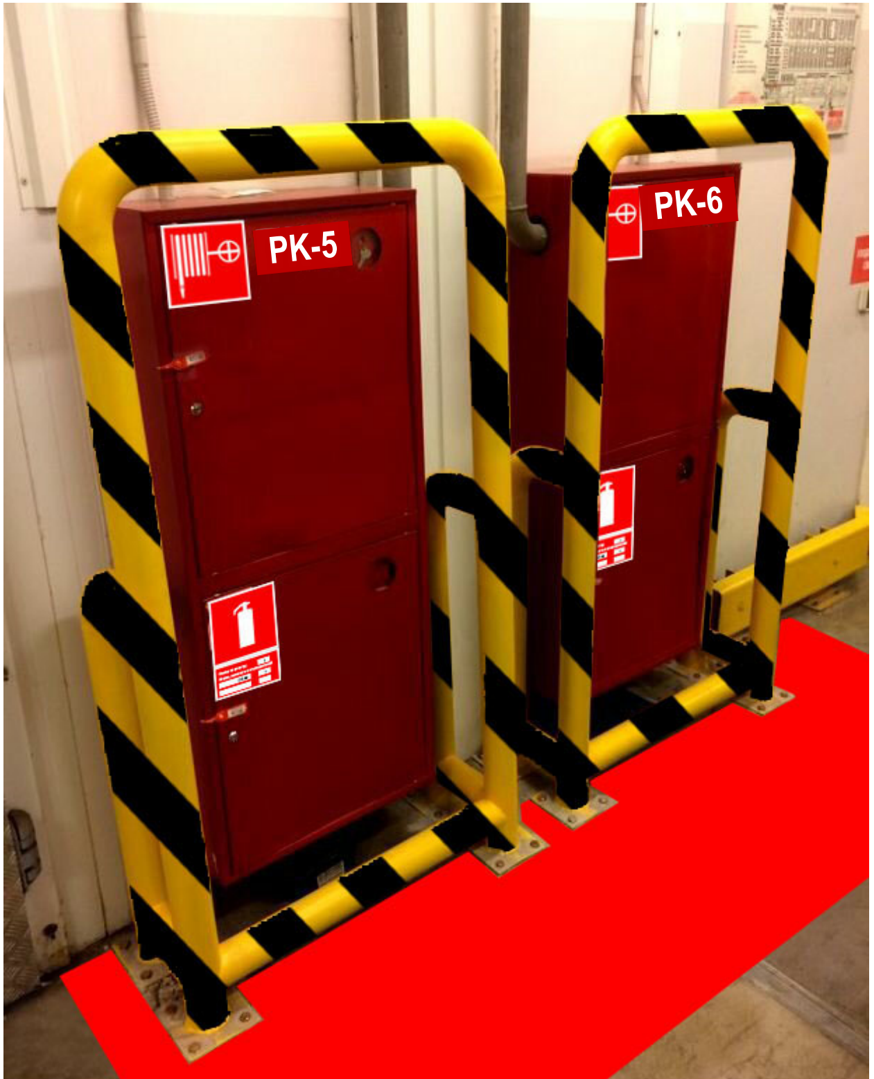
Figure 51 – sample installation of protective structures for a fire hose station
